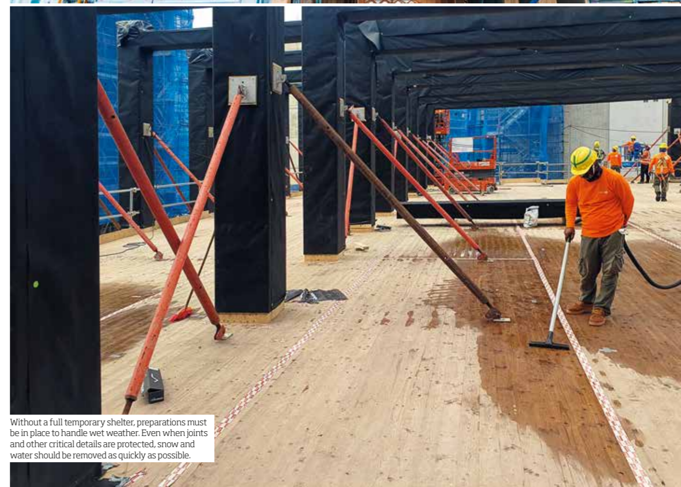
A full temporary shelter provides good protection against moisture-related damage and reduces the risk of the weather disrupting the construction process.
